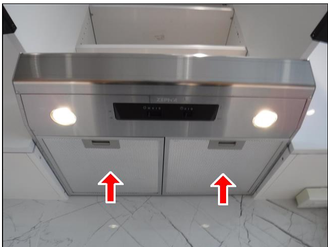
6.0 Item 1(Picture) kitchen exhaust
