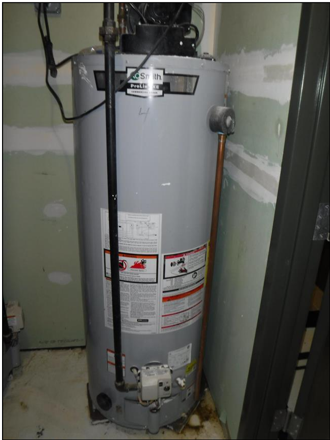
4.2 Item 1(Picture) hot water heater
