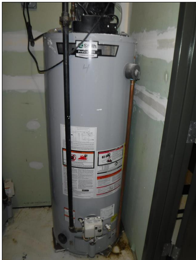
4.2 Item 1(Picture) hot water heater
