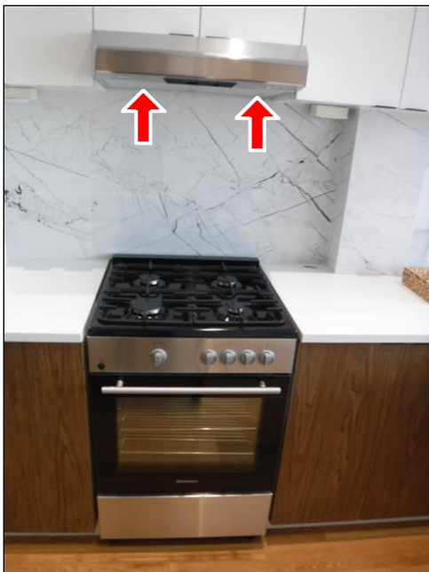
kitchen area exhaust
