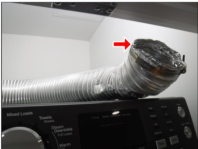
8.3 Item 1(Picture) Dryer flexible vent pipe
