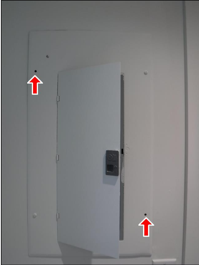
5.0 Item 1(Picture) sub panel in apartment
