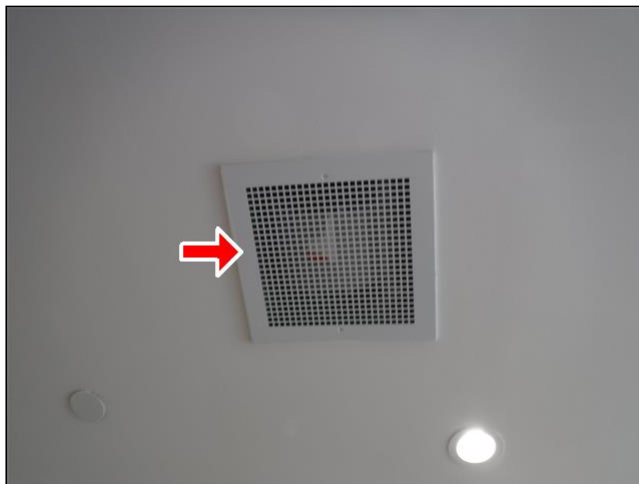
kitchen area exhaust
