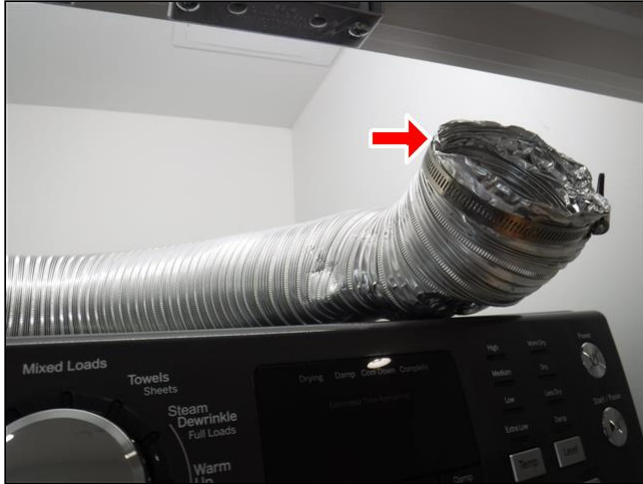
8.3 Item 1(Picture) Dryer flexible vent pipe
